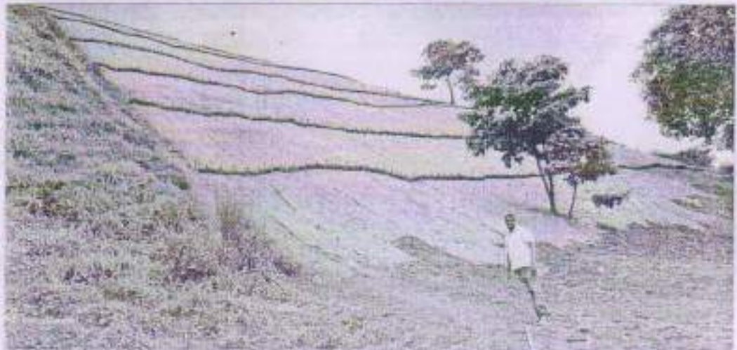
Fixing of Jute geotextiles & Coir logs for ash sliding control and compaction of site for plantation
